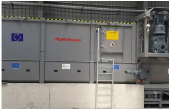
Nabatiyeh MSW treatment plant
