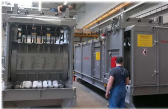
Installation at RRR Kirkouk MSW treatment plant - Iraq
